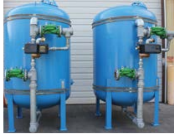
Twin 60"x60" Progressive Flow Water Softeners with 4" service valves and Fleck 3150 regeneration valves.
