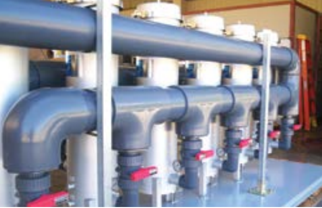
Custom skid mounted pre-plumbed cartridge filter system.
