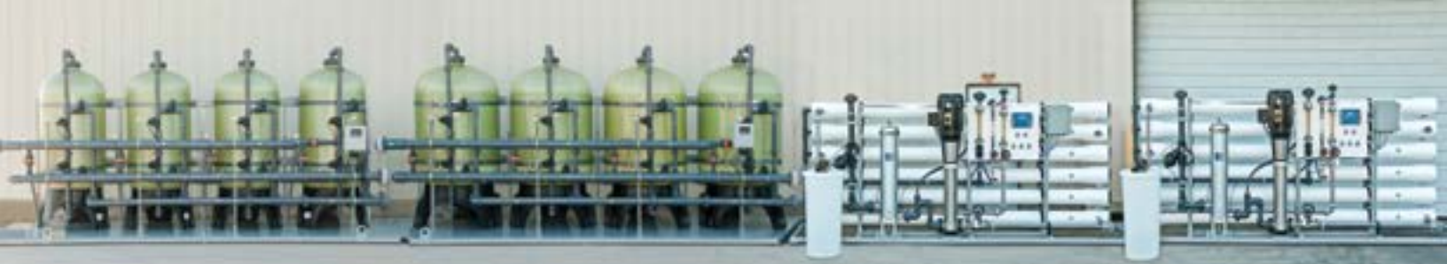
Custom system for distillery. Quad Micro-Z and Quad Carbon systems. Dual RO with a production of 110 gpm each operating at 380 volts, 3-phase, 50 Hz. with Antiscalant chemical feed.
